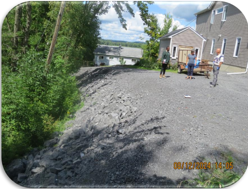
Pre-consulting and inspecting a slope stabilization project Township of Alfred and Plantagenet
