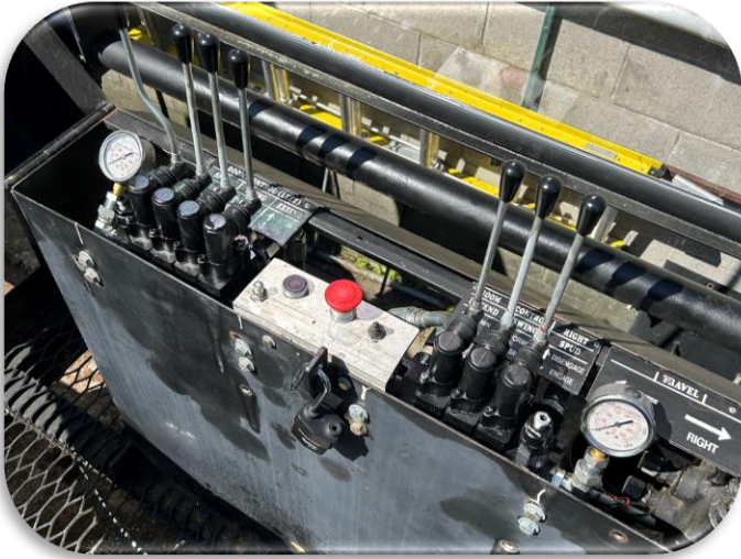
New control panel, Chesterville Dam
