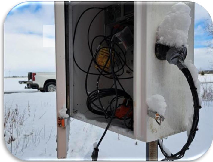
Pleasant Valley Station – as found by SNC staff
