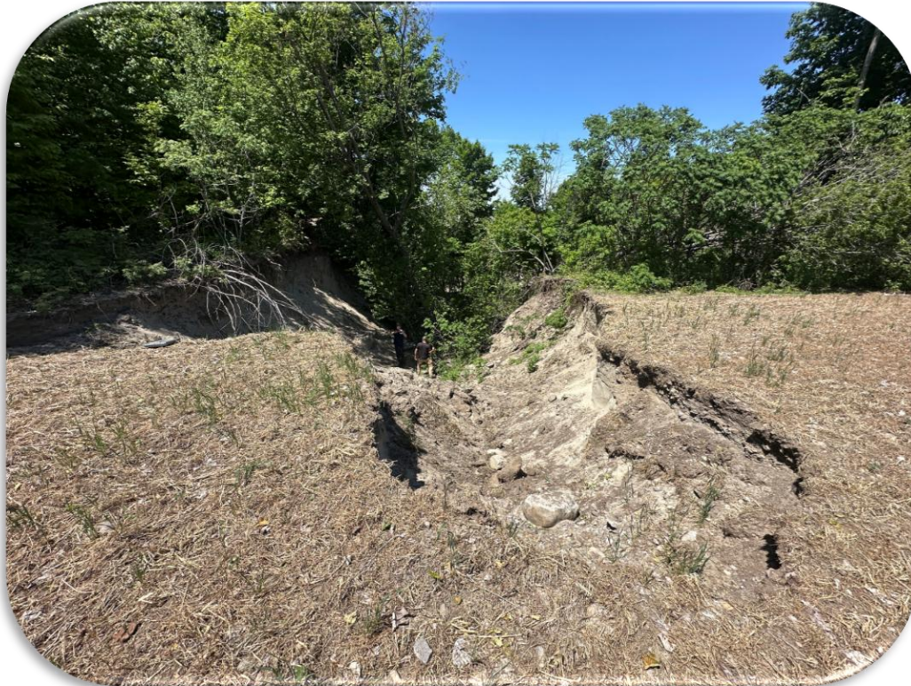
Severe gully erosion in a fine-sand soil type
