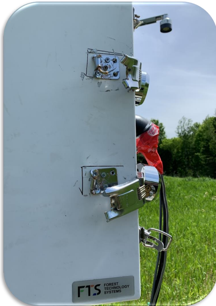
Mill Run telemetry box with damaged HD latches
